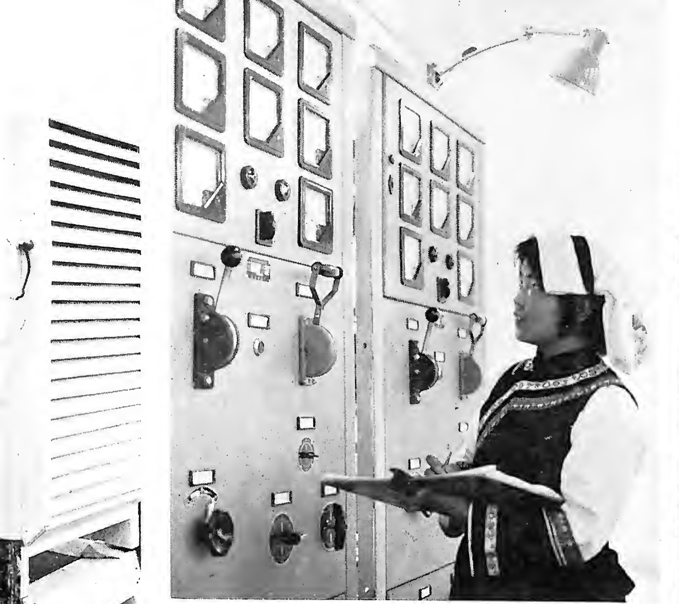
Operator of Yi nationality in the Haiwan Power Station.
